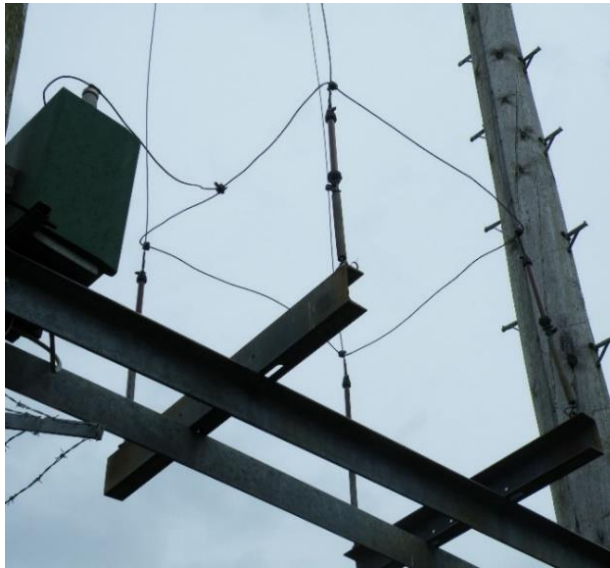
Figure 7. Lacock MF antenna termination. Photo: Mark Carver
